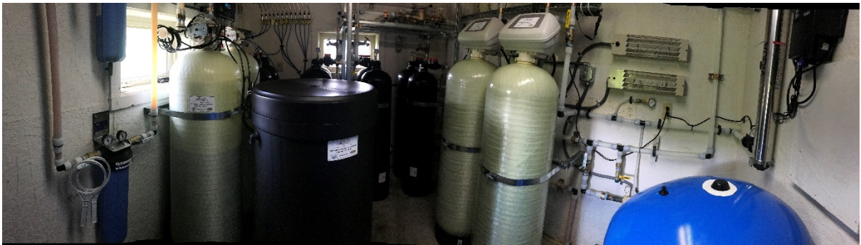
Exhibit 2-3: Installed point of entry treatment system
